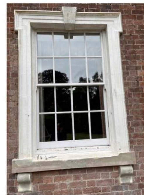
Photograph of one of the new sash windows into an existing sash box frame for the front elevation, ground floor. Only the front elevation of the main house has been done currently.
